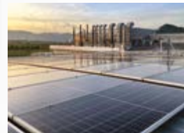
SOLAR POWER PANELS UNDERUTILISED
