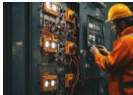
MACHINERY WEAR AND TEAR
