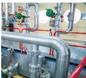
PUMPS, IRRIGATION AND PIPING
